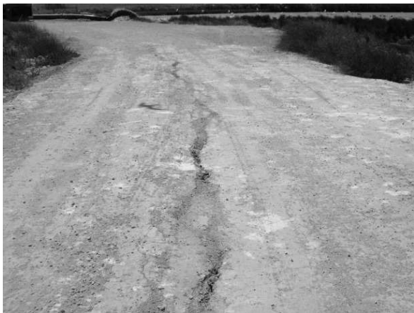
Narrows Bund cracking down the centre of the wall. The edges are also at risk of collapsing. 5 February 2009 Lesley Fischer
